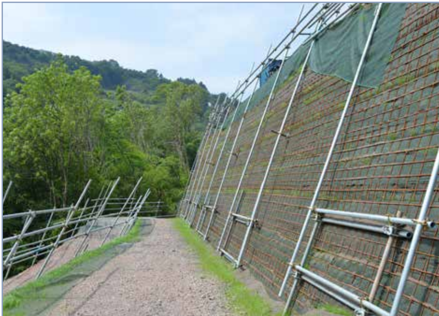
■ Textomur at the A465 Heads of the Valley project in south Wales
