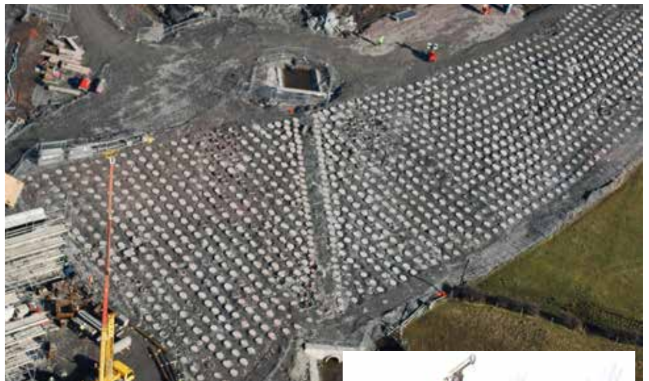
■ Driven cast insitu piles supporting an embankment on the M80 in Scotland
